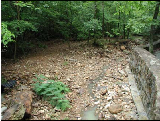
Cedar Branch before construction. High shear stresses were exposing the footers of the rock wall.
